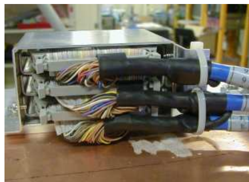
Fig.6b. Cables fixation with the cable tie at the AFEB stack assembly strain relief bracket.
