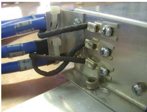
Fig.6a. Ground lug connection to the AFEB stack assembly.
