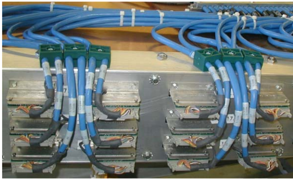
Fig. 5. A view of the anode front-end boards installed on a chamber. Also shown are the AFEB-ALCT cables.
