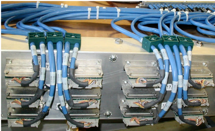
Fig. 5. A view of the anode front-end boards installed on a chamber. Also shown are the AFEB-ALCT cables.
